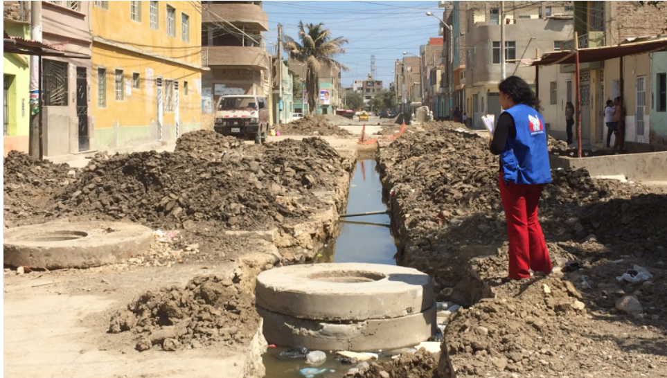
Figure A3 Sewerage project halted
