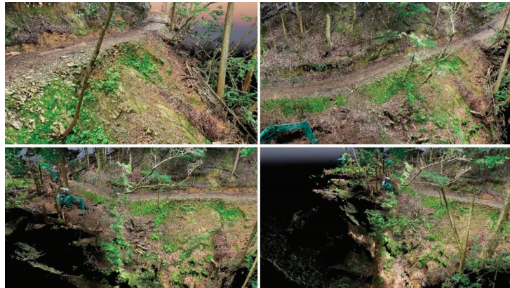
Figure 1. A 3D model generated by SfM analysis before the repair work started.
