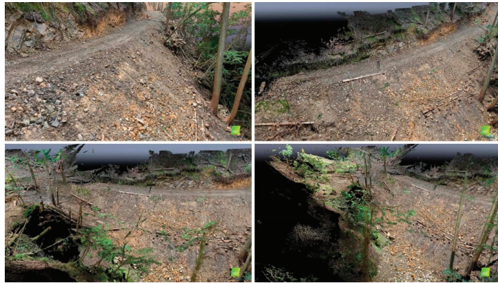
Figure 3. A 3D model generated by SfM analysis after the repair work completed.
