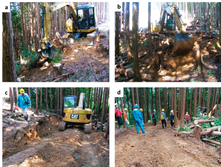
Figure 3. Example of spur road construction in Kochi University Forest during a training course. The excavator dug over the soil for extra depth (a). Then, the loose soil was mixed using the bucket, spread over the designated road width (b), and compacted by the crawler (c). The compaction was carried out for a few layers with a thickness of 20–30 cm each up to the level of the existing road height (d).
