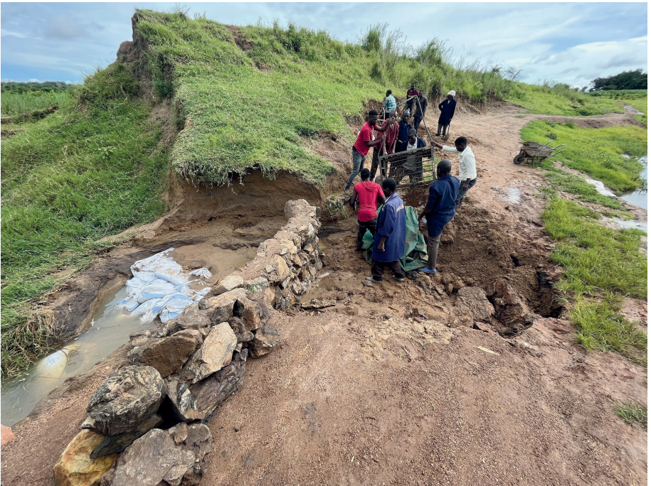
Figure 17: Locals repairing the bridge after the second collapse in February 2023 / Source: Chingalire 2023
