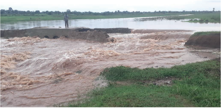
Figure 16: The first collapse of the rural bridge was in January 2023 / Source: Chingalire 2023
