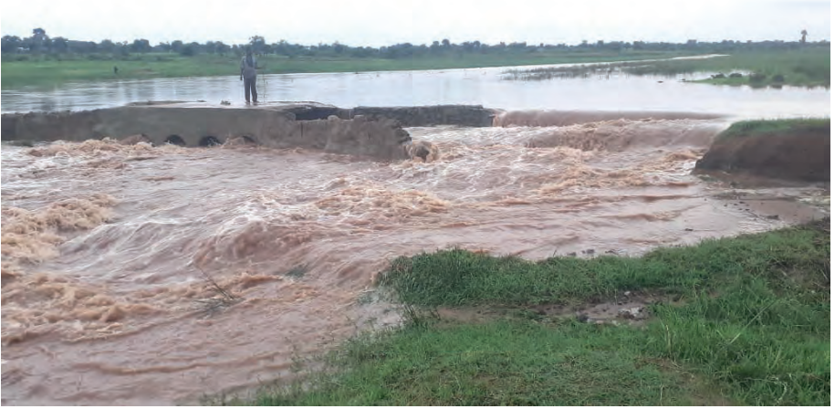
Figure 16: The first collapse of the rural bridge was in January 2023 / Source: Chingalire 2023
