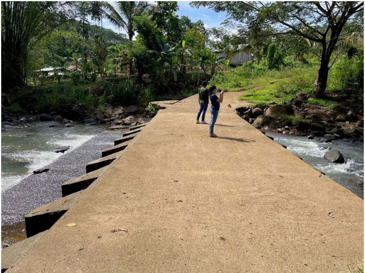
Figure 4. The intended location of the Box Culvert FMI in Lapuyan, Zamboanga del Sur
