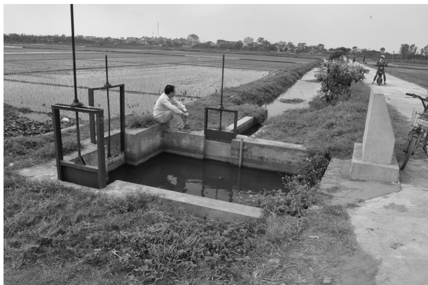
Figure 3.4 Water division work with sluice gates for block rotational irrigation. Source: Photo by S. Yonemura.
