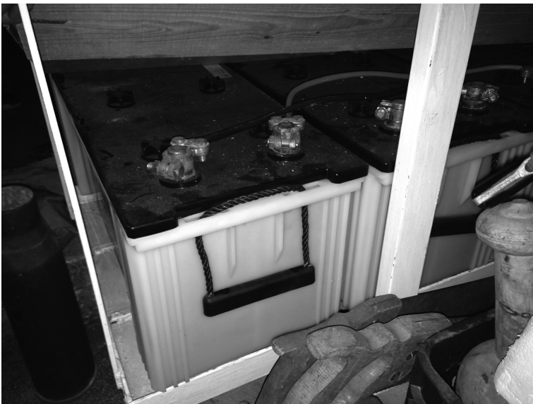
Figure 2.2 Lead-acid batteries mounted on a cradle in the attic of Layla’s house.
