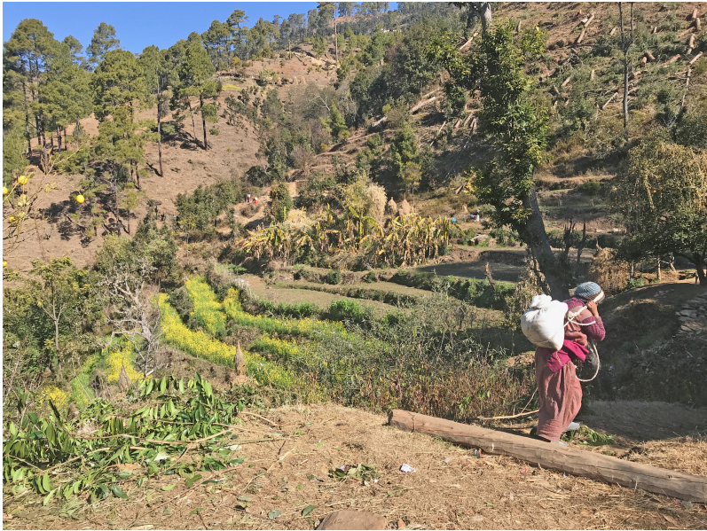
Figure 1.3 A female wage laborer carrying sand to build a new irrigation pond in the village Syauke, Dadeldhura, Nepal, in February 2020 shortly before the corona lockdown (Stephanie Leder).
