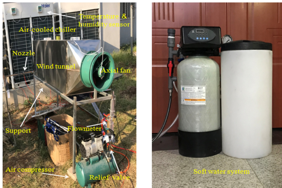
Fig. 2. Photographs of the spray cooling for air-cooled chiller system and soft water system.
