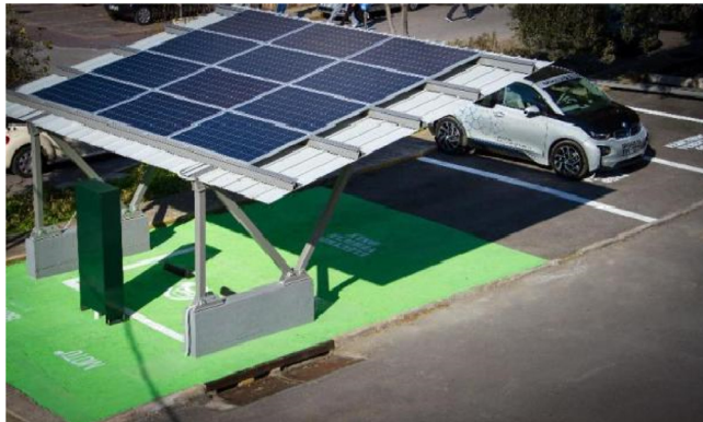
Fig. 6. The autonomous/grid connected solar EV charging station of the SEALAB of the UNIWA.
