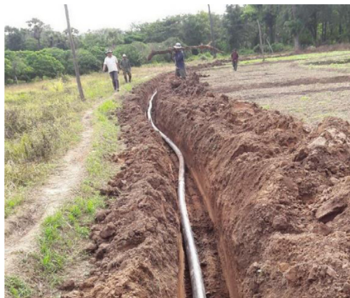
Fig. 4. Main biogas pipeline placed beneath the soil surface.
