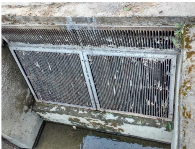
Fig. 4. Typical micro-hydropower trash rack in Nepal.
