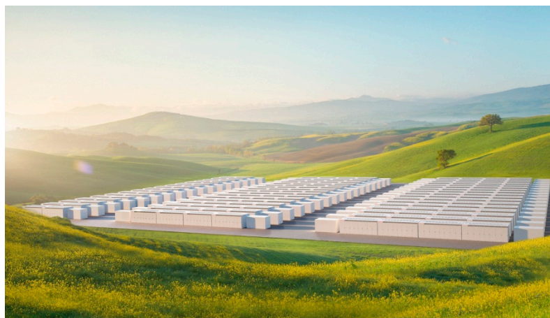
Figure 1. Tesla and Pacific Gas & Electricity Solar & Wind Energy Storage Megapacks at Monterey, California.
