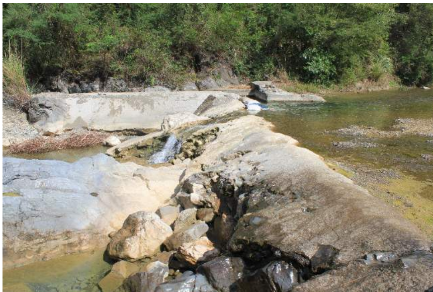
Figure 1A-36. The Parang-Bugnan CIS dam; the damage at the ogee spillway exposes the dam core made of rocks and boulders; the sediments are almost at the dam crest level
