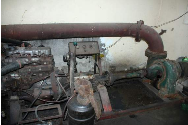
Figure 1A-8. The 8-in dia. centrifugal pump powered by a 4DR5 diesel engine of the Sapa-San Vicente PIS
