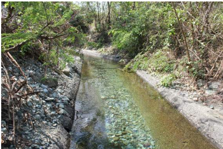
Figure 1A-33. The trapezoidal main canal; the canal bottom is filled with small rocks
