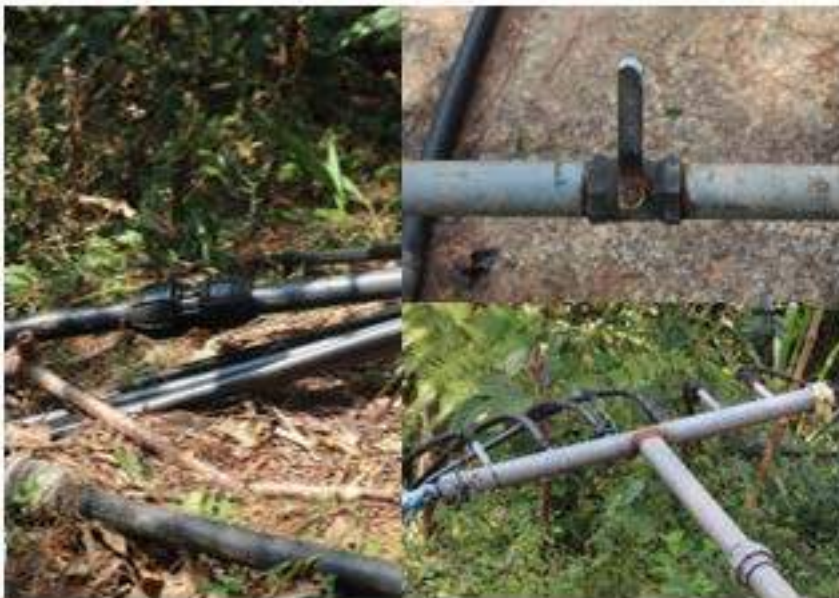
Figure 1A-85. Sample of the union patents, gate valves and improved distribution assemblies of the Taloy Sur CIS
