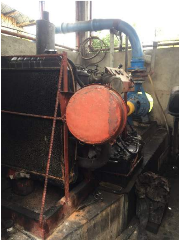
Figure 1B- 35. The centrifugal pump and the diesel engine of the Sigma Sur PCIS
