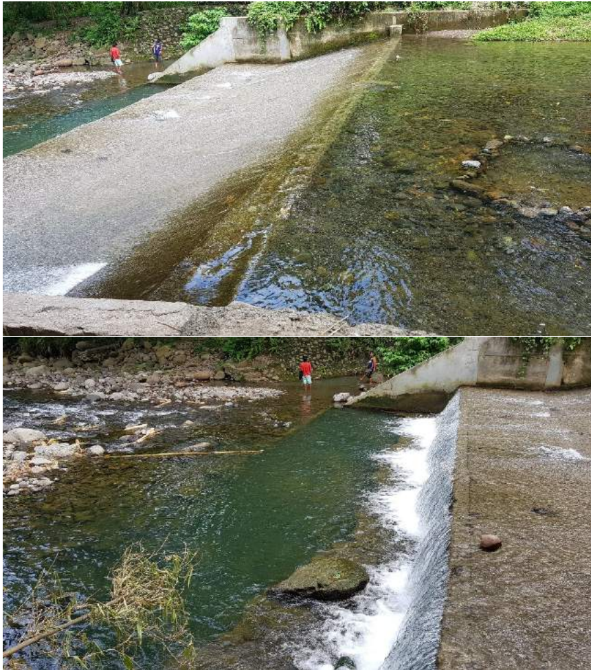
Figure 1C-1. Marapangi Dam of Unifarm CIS showing sedimentation and damaged downstream apron of the dam
