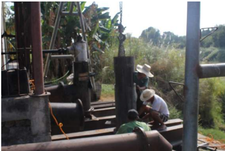
Figure 1A-1. The two 16" dia. mixed flow pumps (one is being repaired); at the foreground is the 10" dia. pipe of the submersible pump
