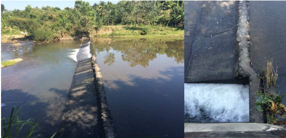
Figure 1A-74. Left: Boliwao dam with high level of siltation; Right: sluiceway
