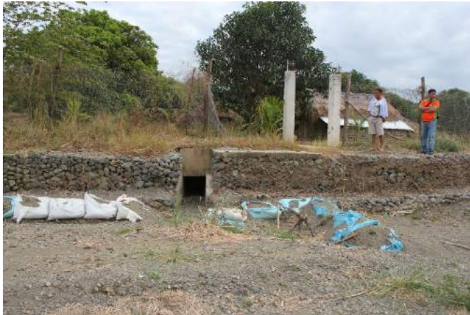
Figure 1A-24. The intake gate upstream of the dam use wooden slabs as gates; the gabions serving as side embankments of the dam are damaged; sand bags used to divert the depleting water last cropping are also shown
