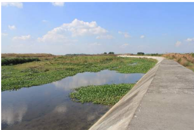
Figure 1A-15. The concrete embankment at the approach to the dam, again showing heavy siltation
