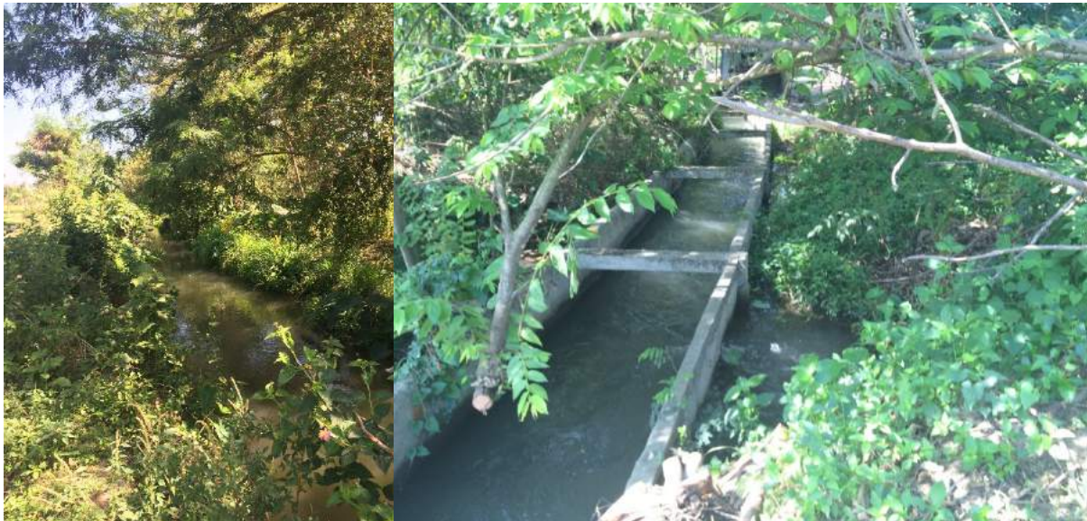
Figure 1A-73. Left: unlined portion of the main canal; Right: lined portion of the main canal with illegal turnout
