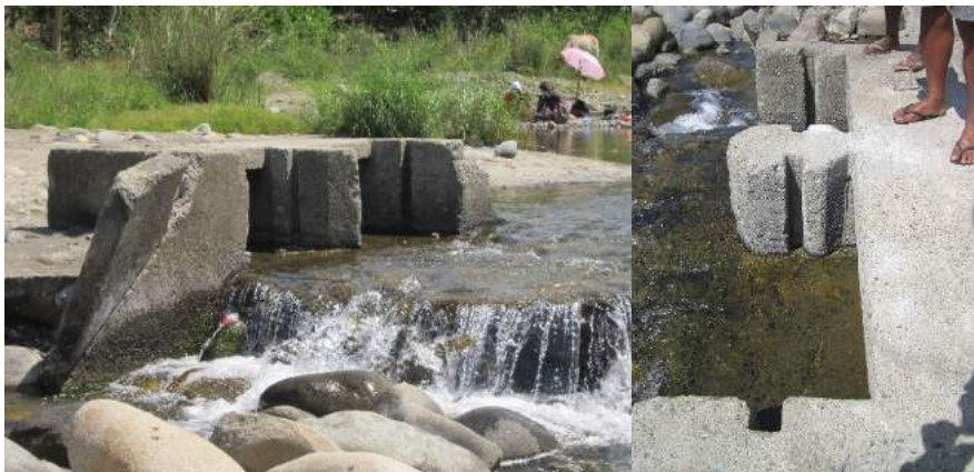
Figure 1A-89. The old intake siphon but was filled with sediments during the typhoons Goring and Iliang
