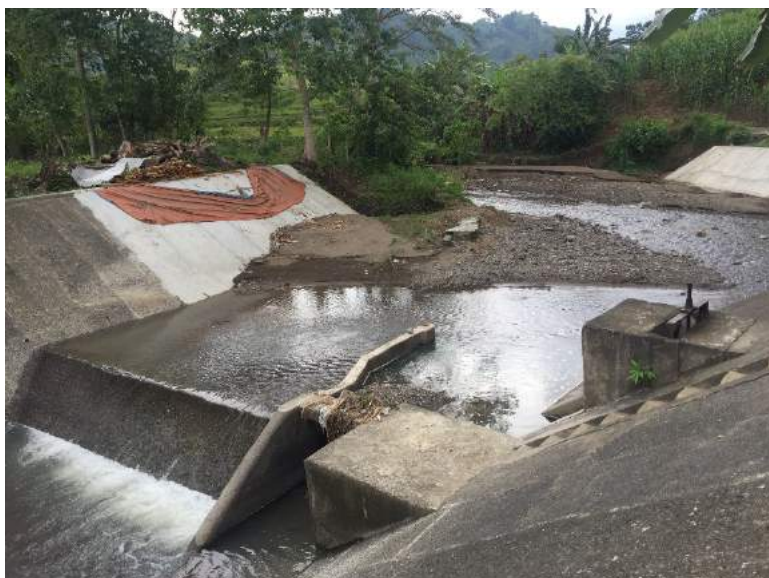
Figure 1C-45. Dam 2 of the system wherein the sand also enters the intake gate
