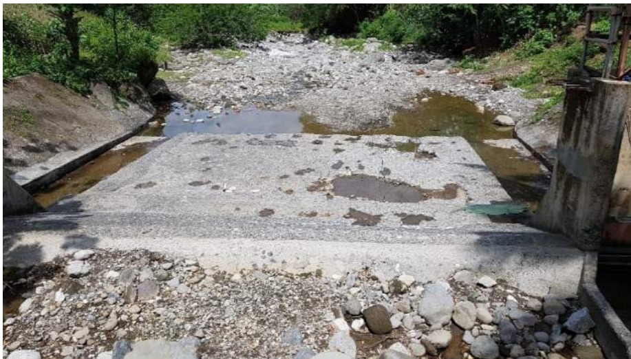
Figure 1C-33. The damaged downstream apron of the dam
