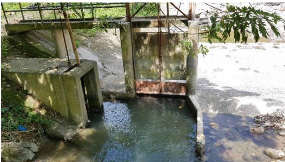
Figure 1C-34. The left sluice gate and intake gate of the dam
