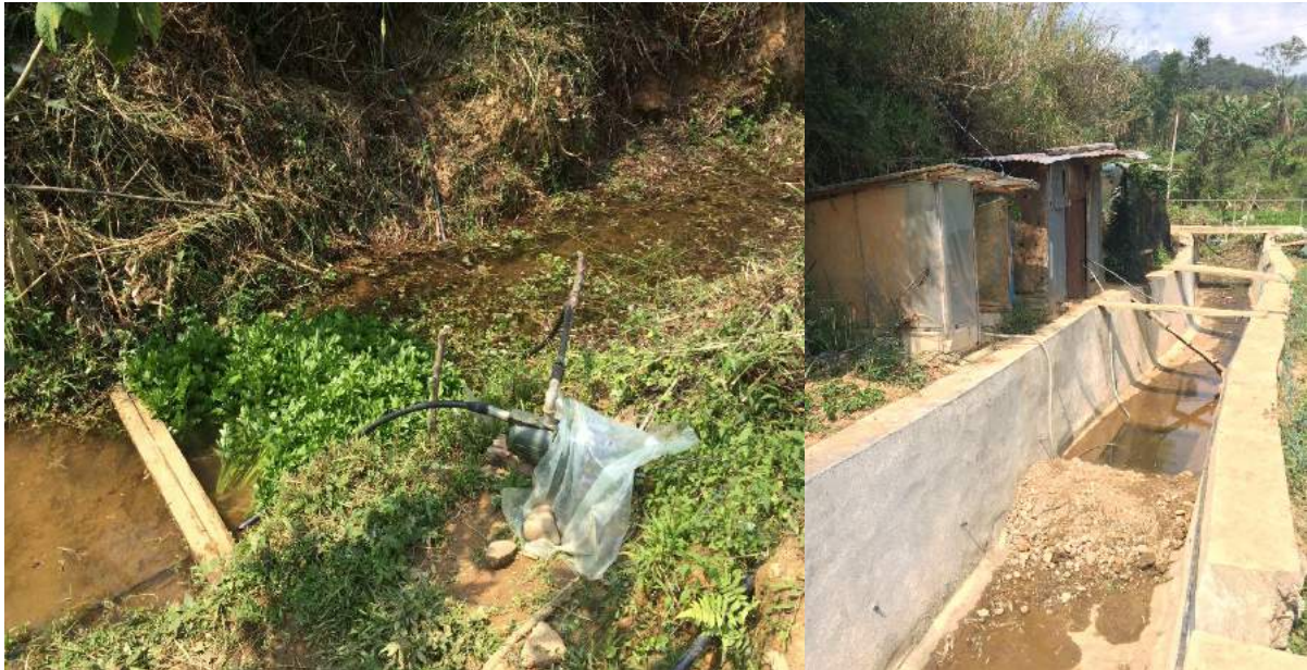
Figure 1A-77. Left: electric motor along the unlined portion of the creek; Right: diesel engines sheltered in pump houses and cavity made by the farmers at the bottom of the main canal
