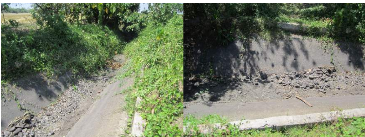
Figure 1A-96. The trapezoidal lined main canal, shown with some sediments at the bottom
