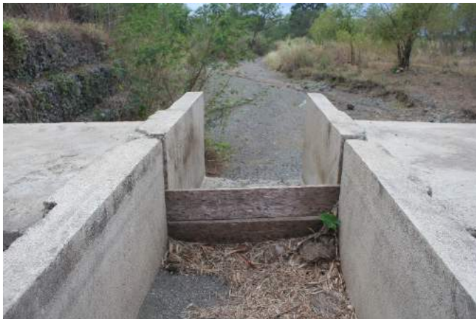
Figure 1A-25. The sluice gate is made of concrete with slots for wooden slabs serving as gates; the background is the downstream portion of the dam
