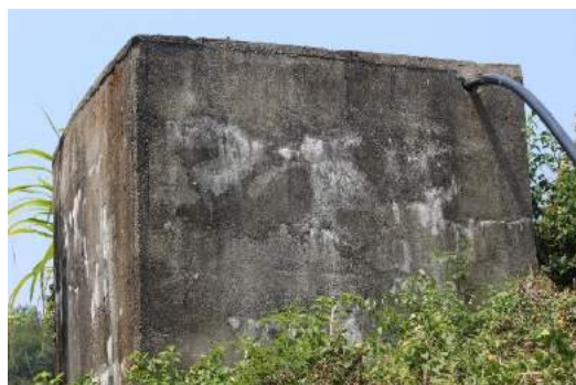
Figure 1A-81. One of several concrete storage tanks showing overflow pipe
