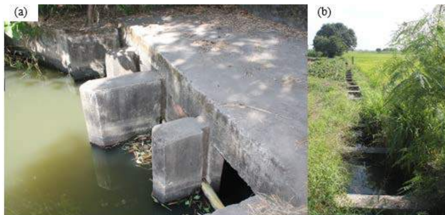
Figure 1A-20. (a) The check gate which the IA refers to as "Dam 2" is used to increase the head at the main canal for distribution to secondary laterals; (b) one of the laterals (concrete-lined) served by the check gate
