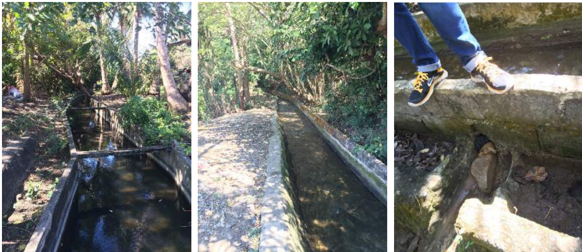
Figure 1A-65. Concrete sections of the main canal upstream (left) and midstream (middle); holes in the concrete canal serving as turnouts for distributing water to laterals; rocks are used to control the flow from the canal (right).
