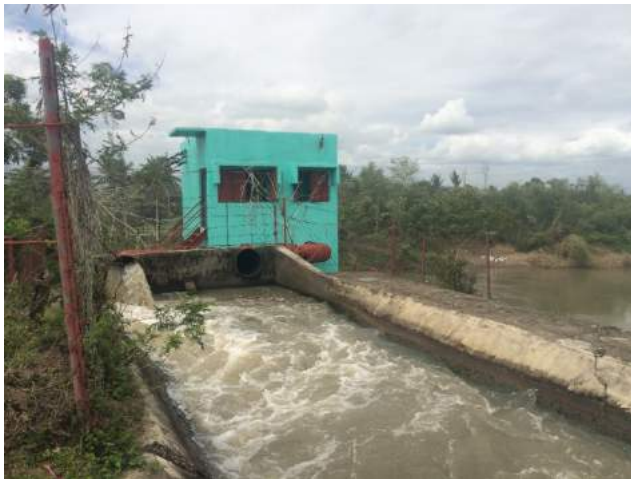
Figure 1A-68. The San Ramon PIS pumping water from the Bicol River; shown here is the discharge from one pump, which is enough to fill the canal to capacity
