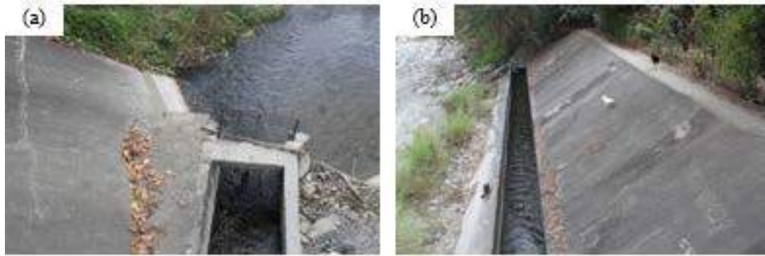
Figure 1A-52. (a) The intake structure with a steel grill to prevent entry of large debris and stones into the main canal; (b) the intake channel at the bottom of the embankment
