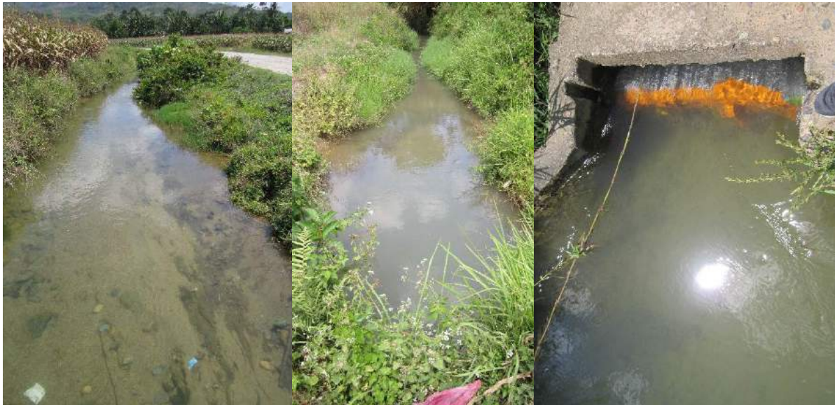
Figure 1A-91. The unlined main and lateral canal and one of the drop structure combined with siphon
