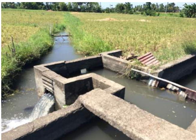
Figure 1A-104. One of the division boxes of the irrigation system with corrugated GI as control gate Source: Author's capture
