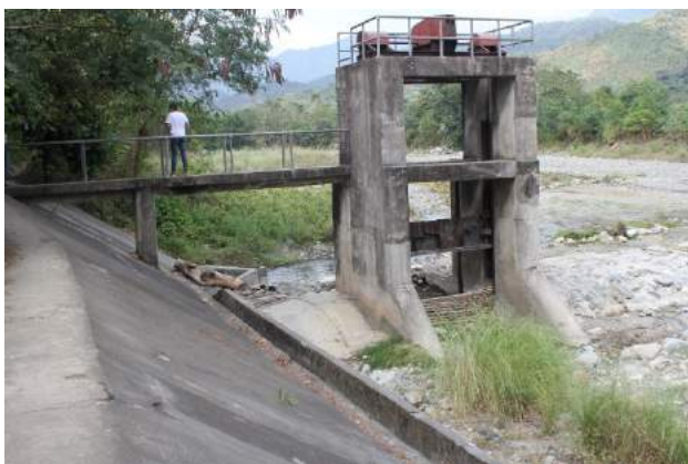
Figure 1A-51. The sluice gate structure and side embankments are still in good condition but the sluice gate itself is now replaced with bamboo and sand bags
