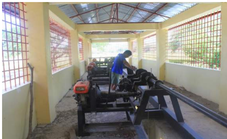
Figure 1A-117. Diesel engines used to control the sluice gates
