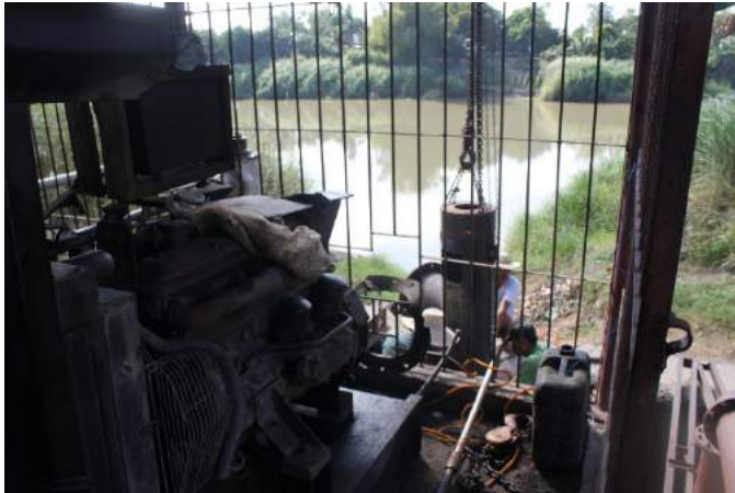
Figure 1A-2. One of 2 Iveco diesel engines for the mixed flow pumps; at the background is the Pampanga River where the PIS derive its waters
