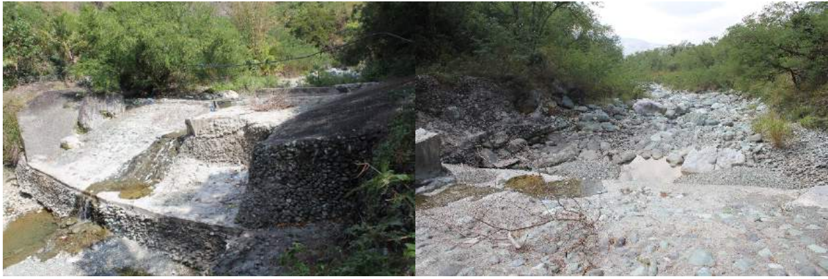
Figure 1A-28. Left: The Inasan CIS dam along the upstream of the Inasan River made of rock and concrete; Right: boulders and rocks downstream of the dam
