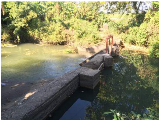
Figure 1A-60. A check gate with one steel gate damaged and replaced with wooden plank
