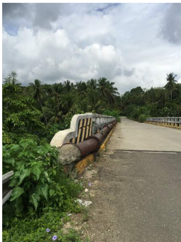
Figure 1B-3. Proposed alternative conveyance to the damaged inverted siphon of Gabayan CIS
