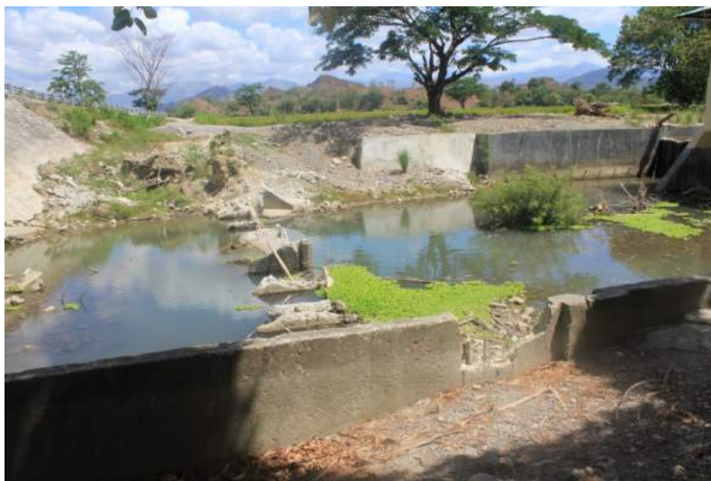
Figure 1A-115. The former Batasan CIS dam that was broken Source: Author's capture
