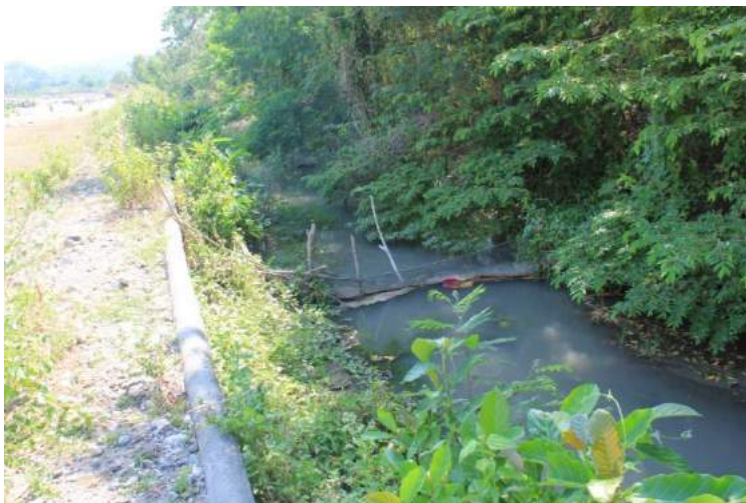
Figure 1A-113. The 2.5-m wide and 3-m deep concrete-lined main canal Source: Author's capture
