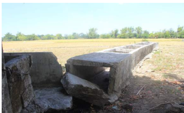
Figure 1A-118. Detached Main canal due to typhoon Glenda
