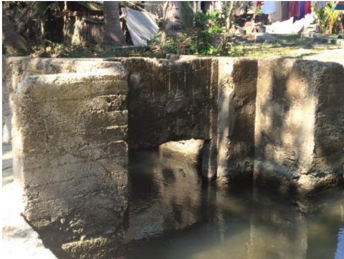
Figure 1A-64. The intake structure with no gate; wooden planks are placed to regulate the flow of water
