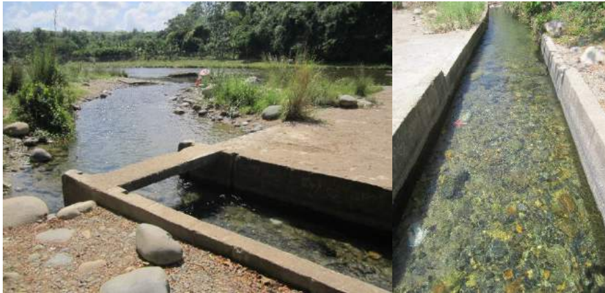
Figure 1A-88. The intake at the side of the dam has no screens and are filled with sediments
