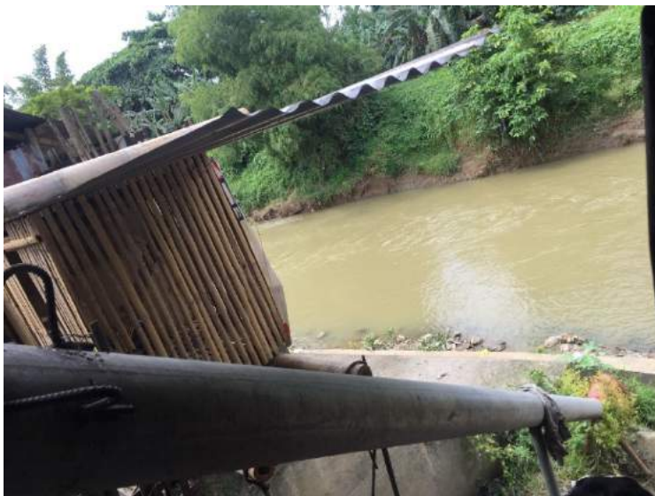
Figure 1B- 34. The 6" suction pipe used in drawing water from the Mambusao River
