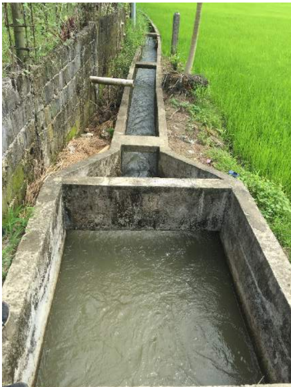
Figure 1B- 36. The main canal of the system as the canal emerged from an inverted siphon across a road
