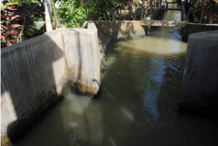
Figure 1A-5. The outlet of the inverted siphon under the road across the concrete sump and pump house; this channels the water into the main canal
