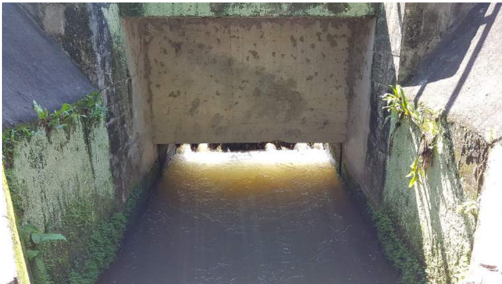
Figure 1C-26. The intake gate that is permanently open Source: Author's capture
