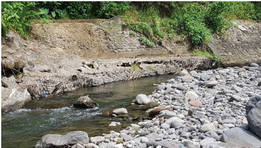
Figure 1C-4. Riprap of bench flume damaged by floods
