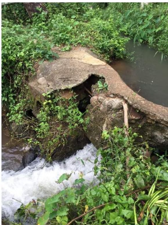
Figure 1C-43. Lateral canal which is broken and no controls
