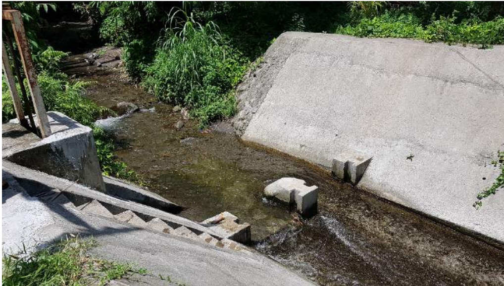
Figure 1C-29. The simple gated dam of Bunao CIS
