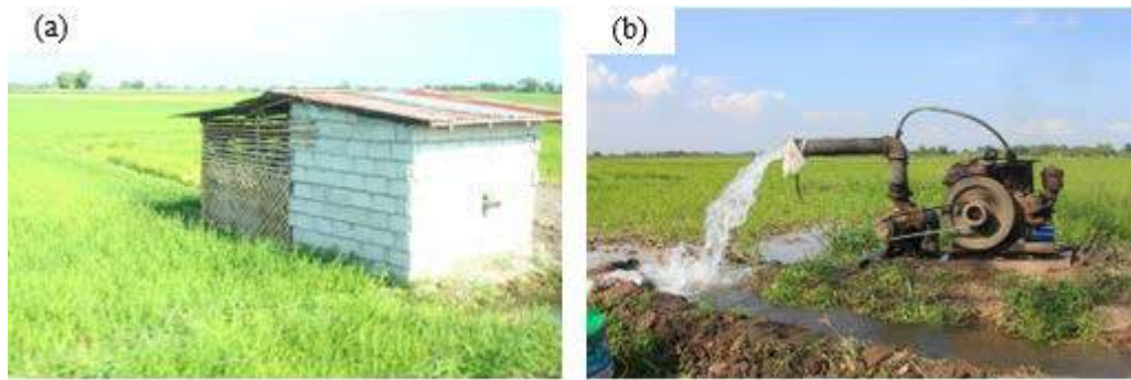
Figure 1A-21. (a) A shallow tubewell (STW) pump house in Anao CIS; (b) an operating STW pump set with a 4-in non-self-priming centrifugal pump driven by a second-hand 9-Hp Kubota water-cooled diesel engine; the discharge was estimated at ~16 lps
