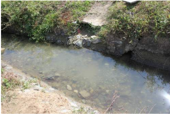
Figure 1A-34. Some portion of the main canal near the highway with damaged side walls and rock laden canal bottom
