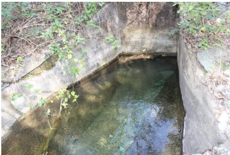
Figure 1A-32. The main canal coming from the underground tunnel from the dam
