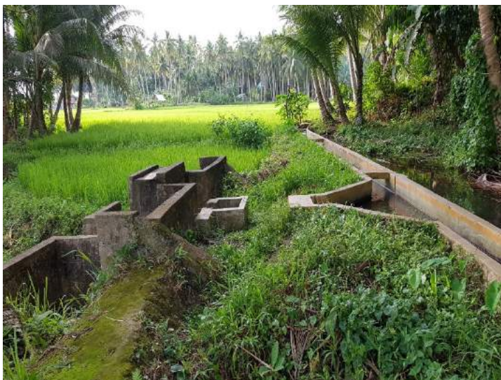
Figure 1B- 10. The original dam constructed in 1960 downstream of the new site. The main canal of the new dam is seen on the right side
