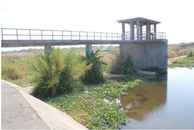
Figure 1A-13. Front view of the Anao CIS showing the heavily silted upstream portion of the dam
