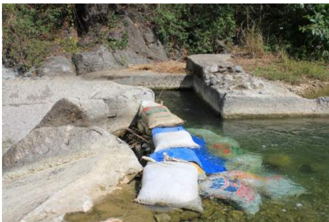
Figure 1A-38. The intake structure showing damaged concrete parts where water flow is guided to the inlet by piles of sand bags Source: Author's capture
