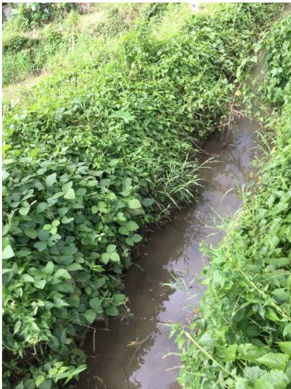
Figure 1C-49. Silted main canal connected to Dam 2 Source: Author's capture
