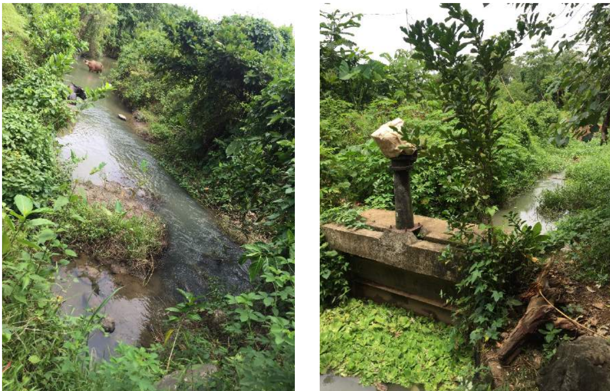
Figure 1B- 30. The unlined main (left) and lateral (right) canal with some control structure
