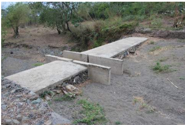
Figure 1A-23. There is no water in the creek during the time of visit and the sediments are almost up to the dam crest
