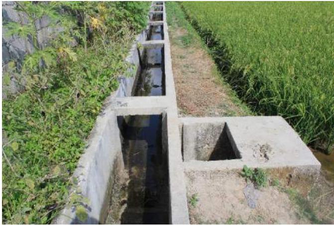
Figure 1A-10. The concrete-lined main canal with a simple turnout gate using slots and wooden slabs as gate
