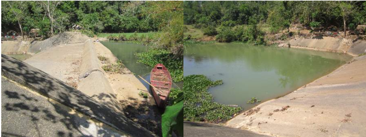
Figure 1A-98. The impounding dam upstream (left) showing crest height increased by a few feet where the overflow water goes downstream (right) to the brush dam
