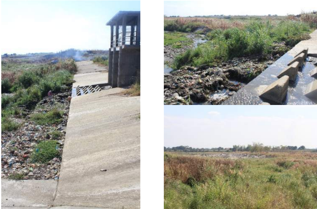
Figure 1A-16. Clockwise from left: (a) scouring at the downstream apron, the sluice gates and intake structures are seen at the middle of the dam; (b) the gabions are damaged and accumulating garbage; (c) the quarry operations just downstream of the dam location
