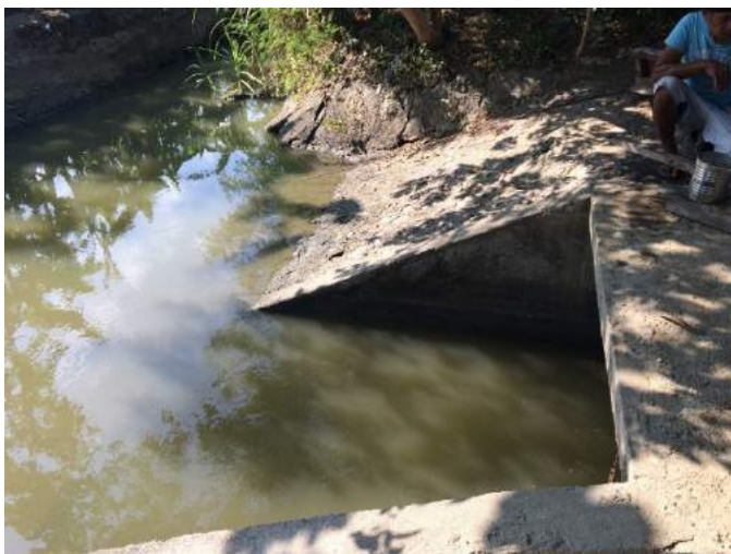
Figure 1A-56. The end of the tunnel connecting the from intake and main canal Source: Author's capture
