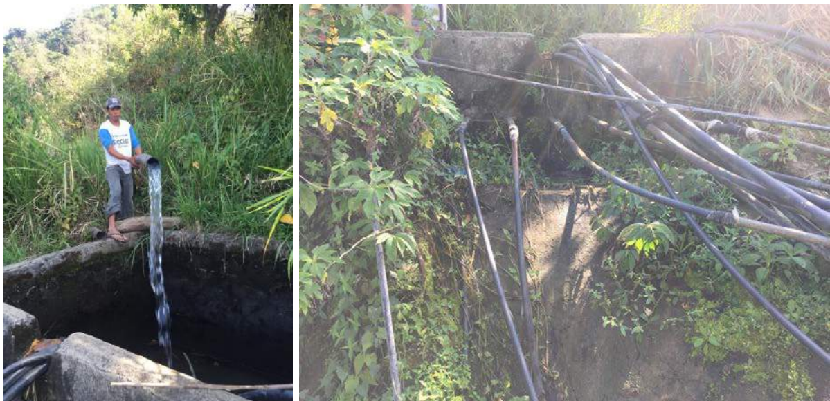
Figure 1A-79. The main tank showing flow of water from the source and the distribution pipes to the other tanks.
