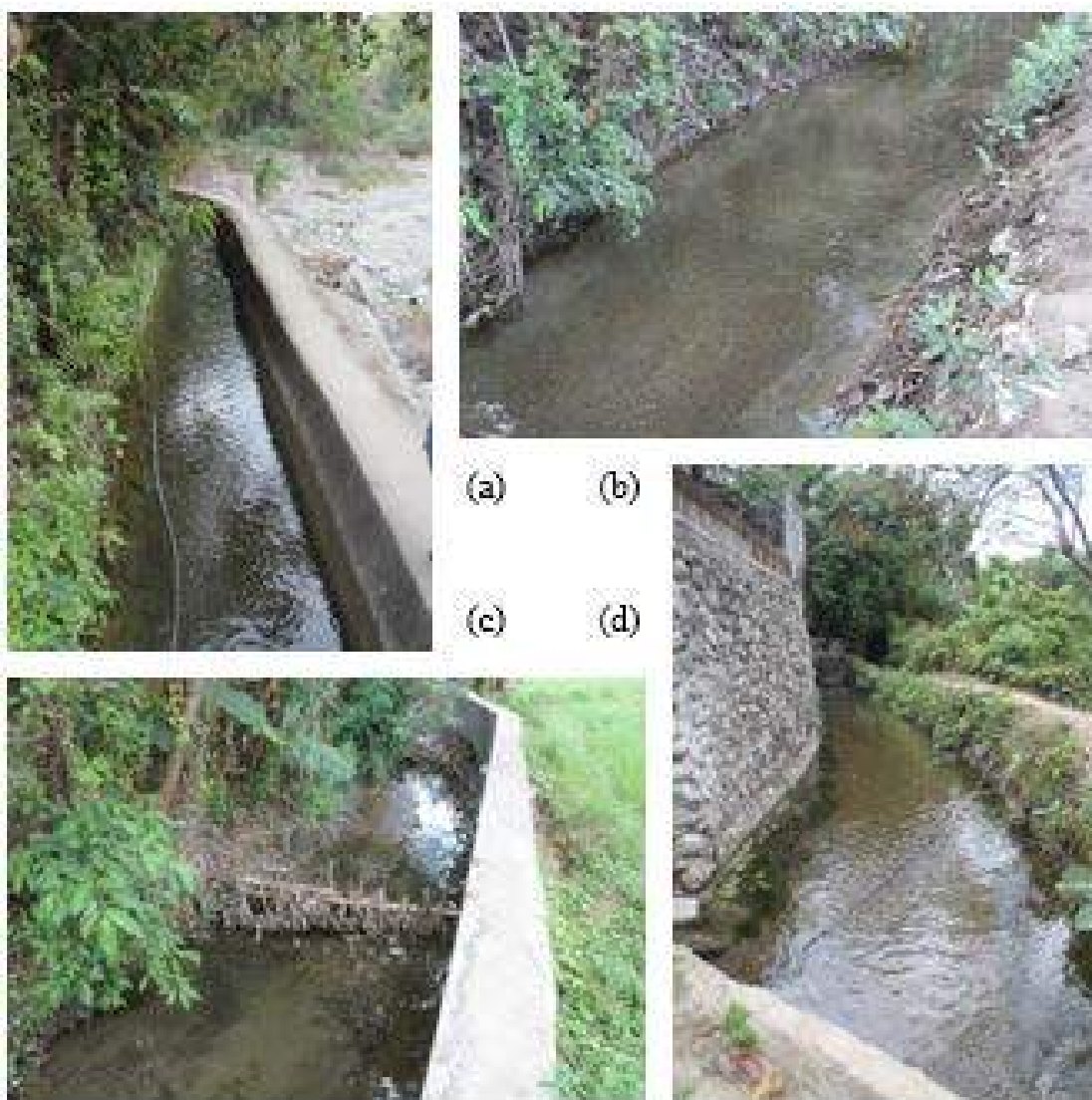
Figure 1A-53. (a-d) Pictures of the canal system with some having concrete lining, some have ripraps and most are unlined; most canals exhibit heavy siltation
