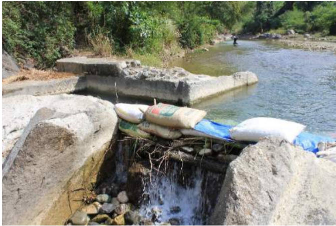
Figure 1A-37. The damaged sluice gate now made up of piled wood, rocks and sand bags Source: Author's capture
