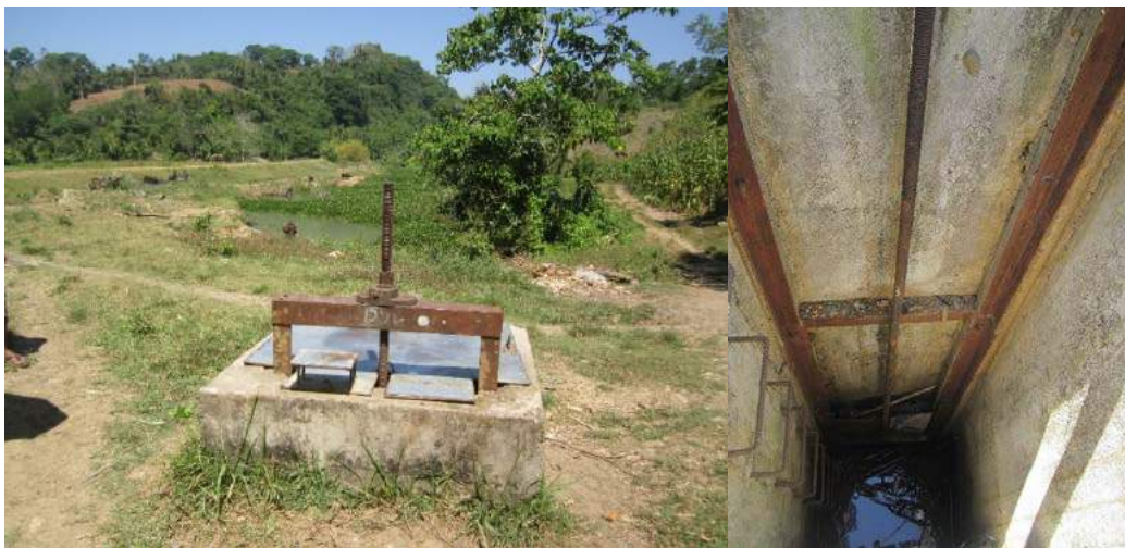
Figure 1A-99. The intake structure with cover (left); the intake gate inside
