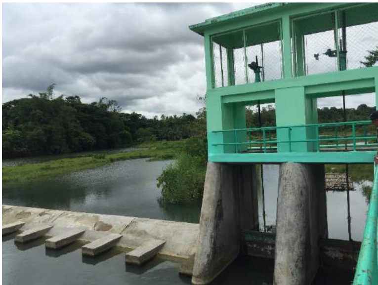
Figure 1B- 14. Two steel gates of the dam which measured 1.5 m each Source: Author's capture
