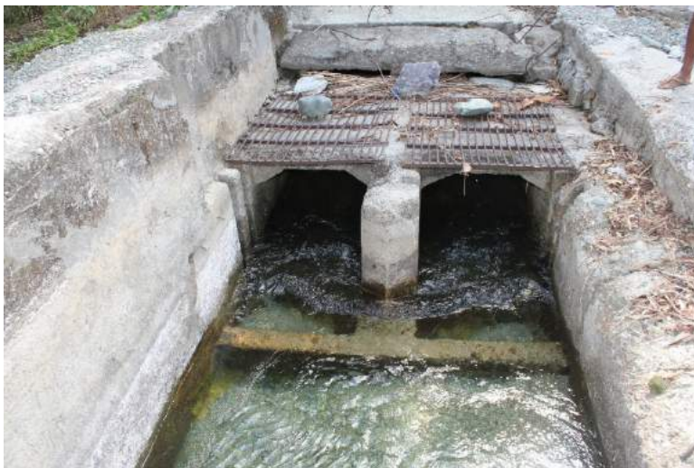
Figure 1A-30. The intake structure leading to the underground tunnel into the main canal
