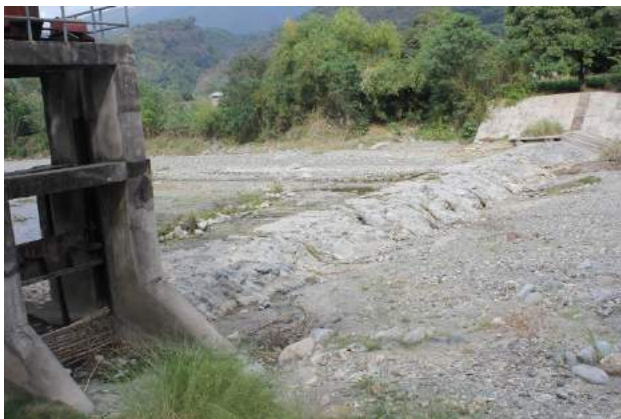
Figure 1A-50. The Ngayao-ngaoan CIS dam showing damaged ogee spillway and silts up to the dam crest; also shown is the sluice gate now made of bamboo
