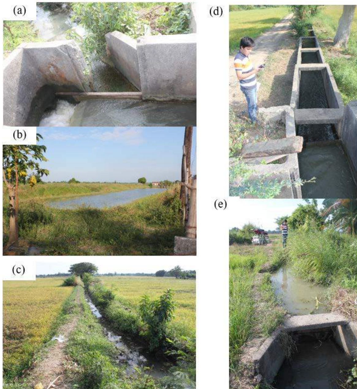
Figure 1A-7. (a) A typical control structure combining a turnout (using wooden slabs), a drop and a road crossing; (b) one of several fishponds being served by the PIS; (c) a typical unlined lateral; (d) continuation of the concrete-lined main canal with control structure combining turnout (wooden slabs) and drop structure; (e) the end check of the main canal, from here on the canals are unlined.
