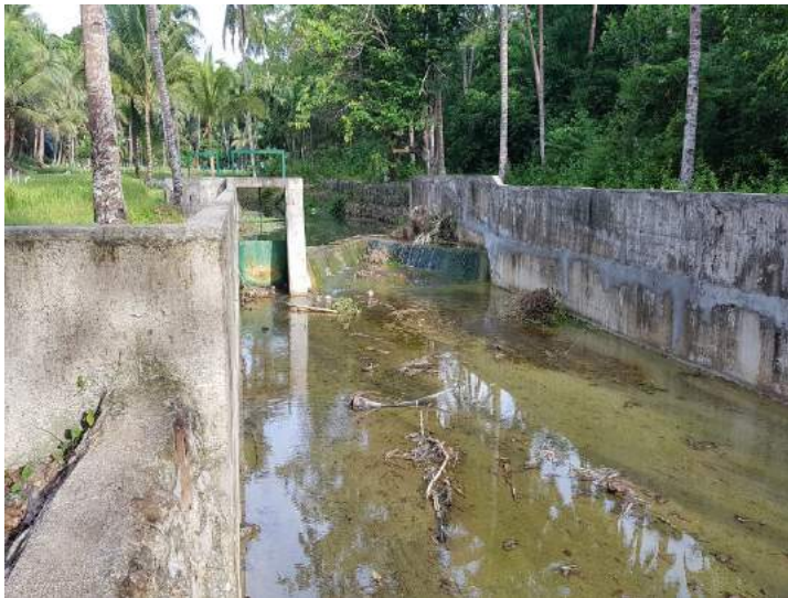
Figure 1B- 9. The new dam of the Maljo CIS constructed in 2012. It is a run-of-the-river type dam with a duckbill crest
