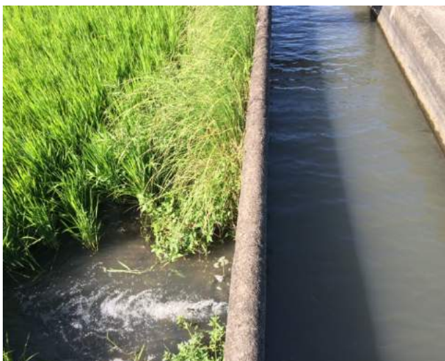
Figure 1A-110. Illegal turnouts directly tapped on main canal
