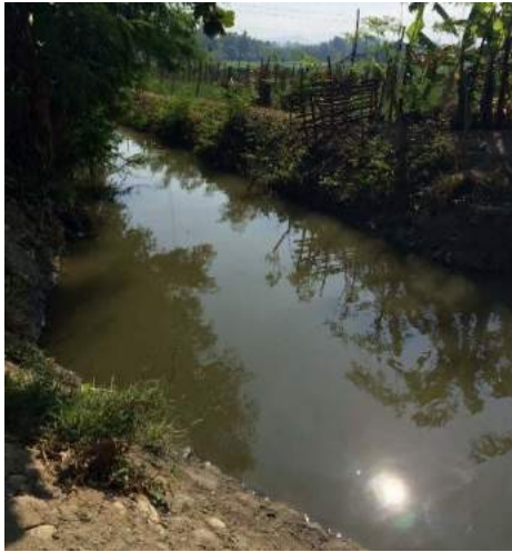
Figure 57. The main canal is unlined and heavy with siltation
