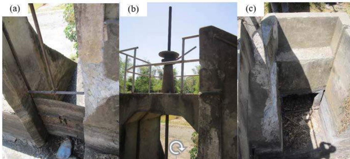
Figure 1A-95. (a) The wooden sluiceway gate; (b) the operating screw of the sluiceway gate; (c) the intake gate with broken regulator
