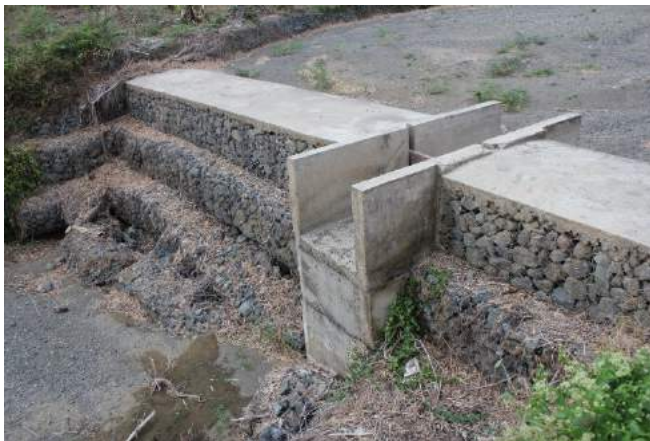
Figure 1A-22. The Cordero CIS dam along Arimal creek is made up of gabions and plastered with cement at the crest; shown at the left side are the damaged gabions where water seeped underneath the dam
