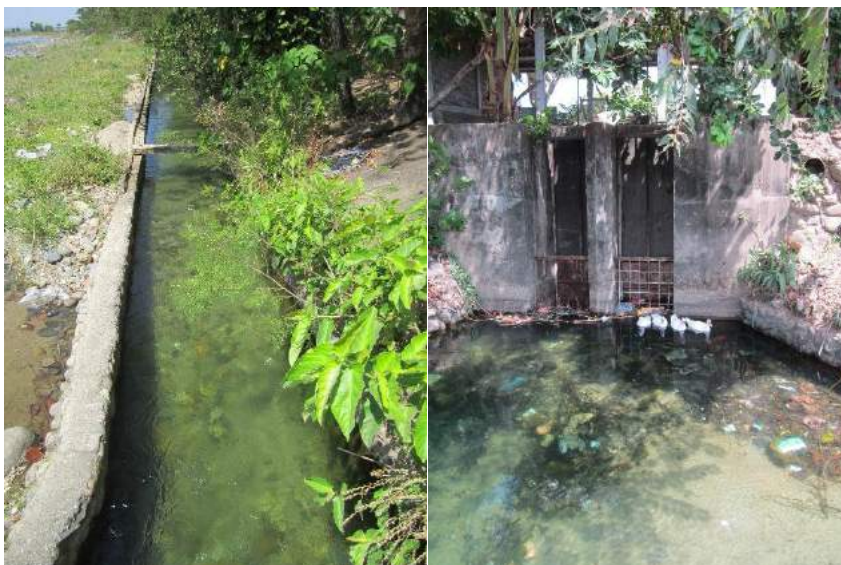
Figure 1A-90. The intake canal filled with sediments and the intake gate where the entry way is also filled with sediments
