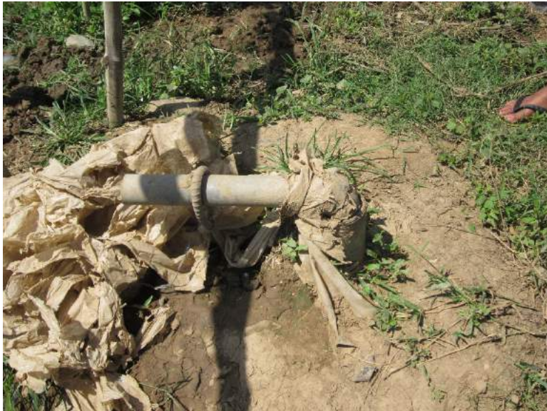
Figure 1A-92. One of the STW units; covered with plastic is the installed 4" PVC pipe, tee and reducer; visible is the 3" discharge pipe where the rubber hose of the pump is attached
