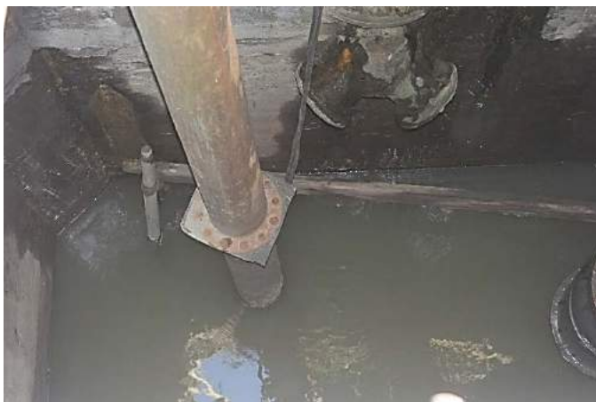
Figure 1A-3. The concrete intake pit for the suction pipes of the Gulap Pump Irrigation System; also shown is the 10-in pipe of the submersible pump
