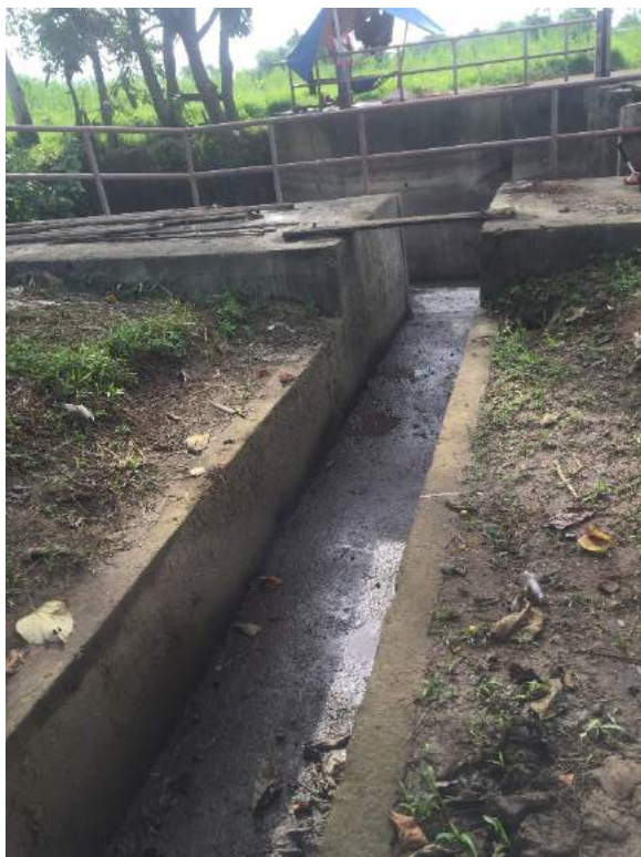
Figure 1B- 18. Intake of Sta. Elena CIS going to the main canal
