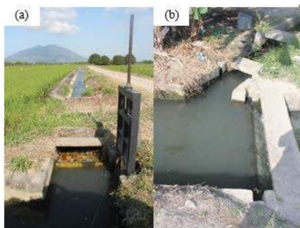
Figure 1A-19. (a) A check gate that serves as a turnout for distributing water to a secondary lateral; (b) a flow dividing structure to a lined lateral; the control has slots for wooden slabs and combined with a shallow drop
