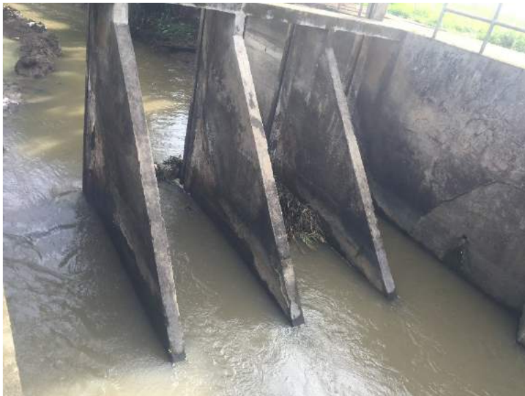
Figure 1B- 17. The buttress dam of Sta. Elena CIS. The IAs use wooden planks since no steel gates were installed
