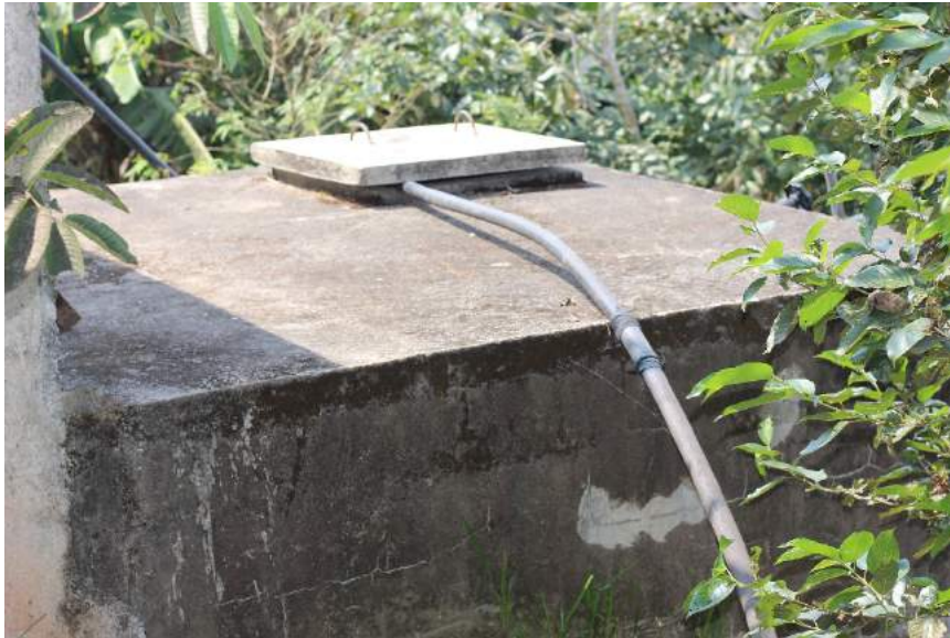
Figure 1A-84. One of the concrete storage tanks of the Taloy Sur CIS showing the entry point for tank cleaners
