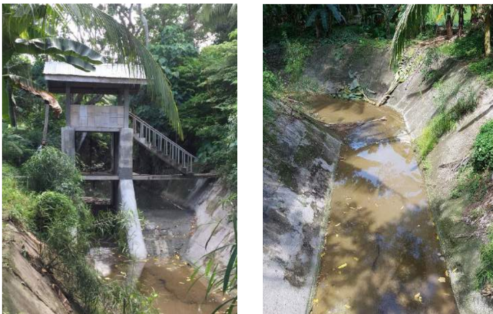
Figure 1C-8. The dam of Butilon CIS with the extended apron and side wall
