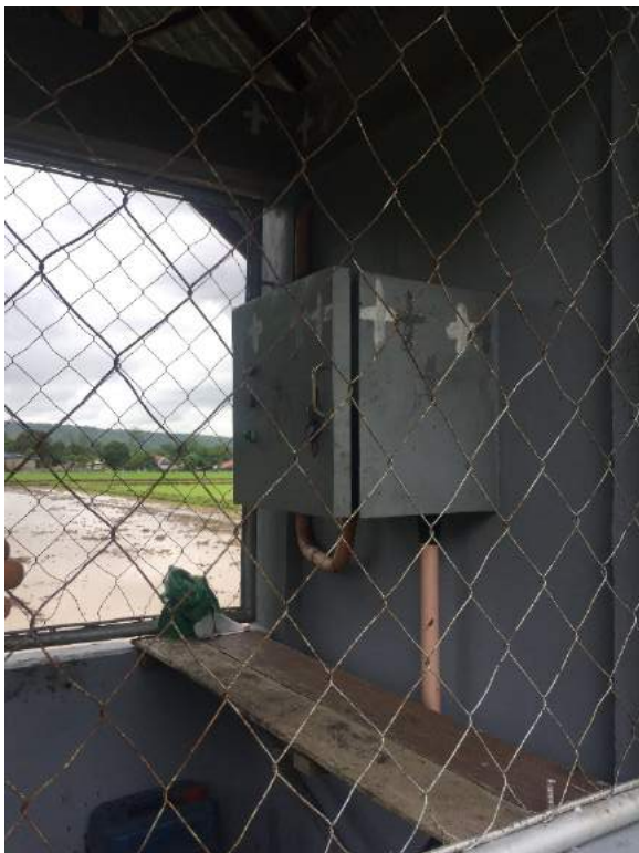
Figure 1B- 23. The transformer for the submersible pump of the CIS
