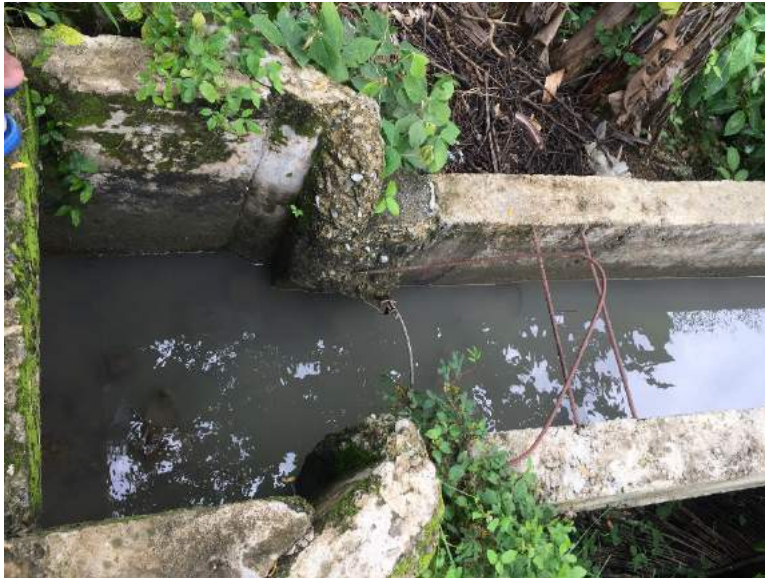
Figure 1B- 28. Connection of the main canal and the elevated flume showing the difference in width and height
