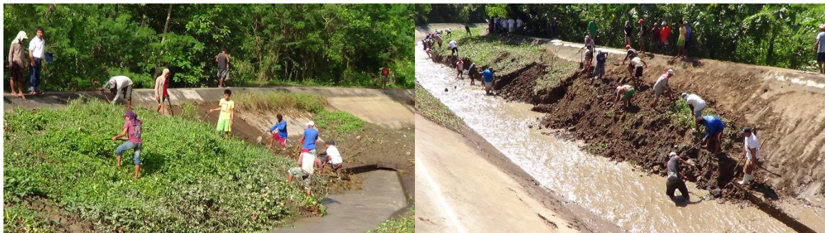
Figure 26. Clearing of the settling basin by combined manual and hydraulic flushing using the silt ejector during the fallow period.
