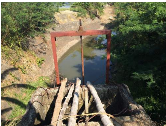
Figure 1A-55. The Baay CIS intake structure Source: Author's capture
