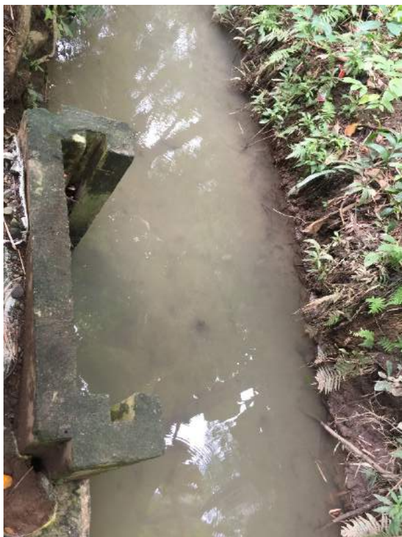
Figure 1C-46. Silt ejector in main canal connected to Dam 1
