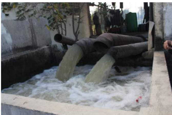
Figure 1A-4. The concrete sump where the discharge pipes of the 3 pumps empty before distribution to the main canal; the middle pump is being repaired; the water is sediment laden
