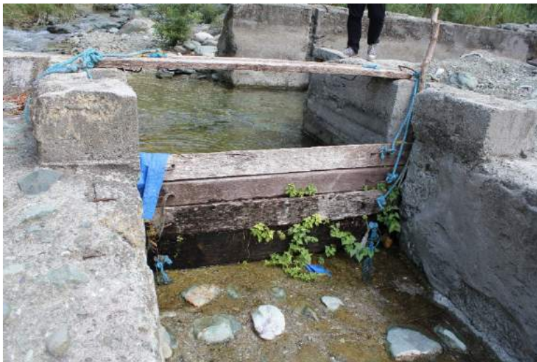
Figure 1A-29. The sluice gate is made of wooden slabs stacked together in a slot serving as water level control gate
