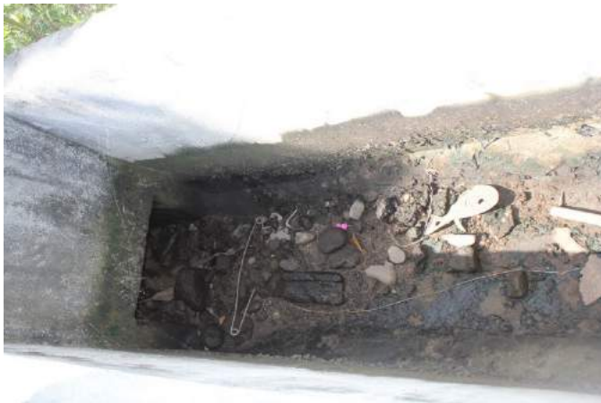
Figure 1A-11. Siltation and garbage observed from the portion of the main canal near the pump
