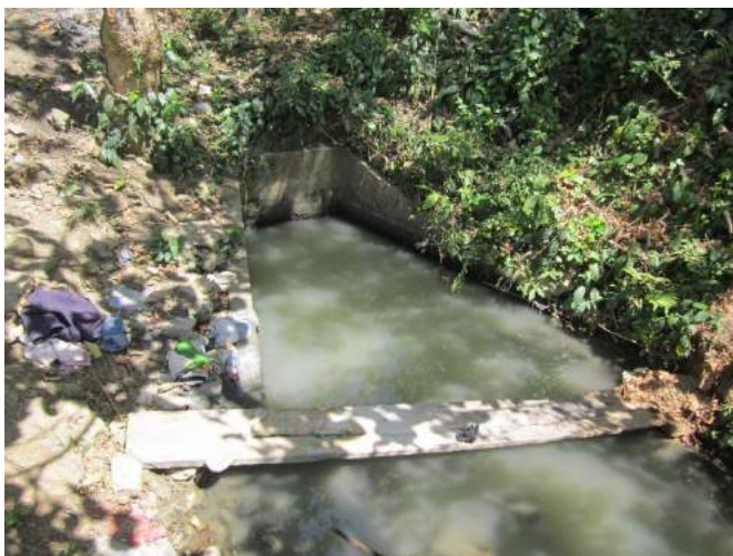
Figure 1A-100. The outlet from the intake gate leading to the trapezoidal main canal
