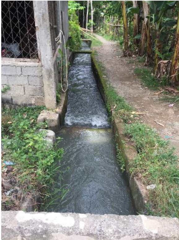
Figure 1B- 11. Main canal of Tagbawto CIS with width of 100 cm and height of 80 cm
