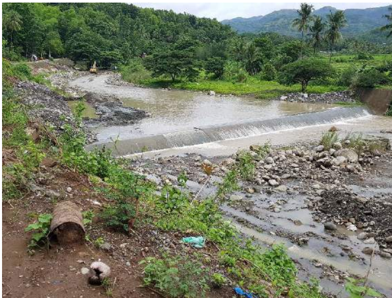
Figure 1B- 24. The Tumagboc CIS dam affected by a road construction on the left Source: Author's capture
