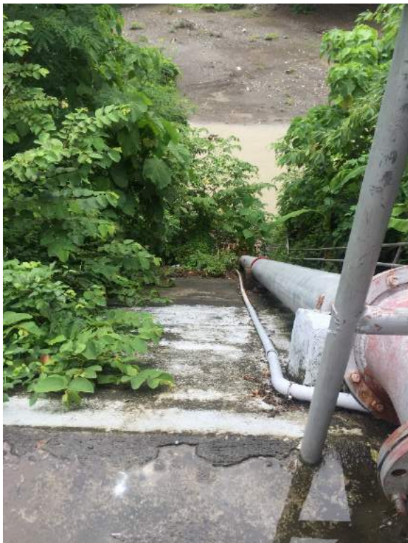
Figure 1B- 21. The 10" pipe connected to the original pump that delivers water to the main canal
