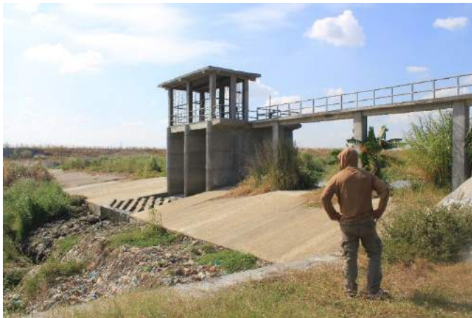
Figure 1A-14. Rear view of the Anao CIS showing the wide dam crest and the damaged and garbage-filled gabion support downstream of the dam
