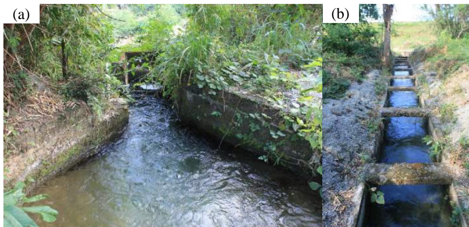
Figure 1A-42. (a) Outlet of the inverted siphon under the river; (b) the concrete-lined lateral canal after the outlet of the inverted siphon used to distribute the water to Parang-Bugnan CIS area across the river
