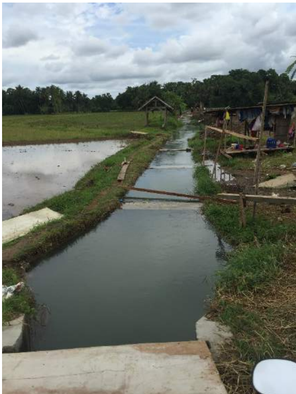
Figure 1B- 12. Ongoing canal construction with width of 2 m and depth of 1.25 m
