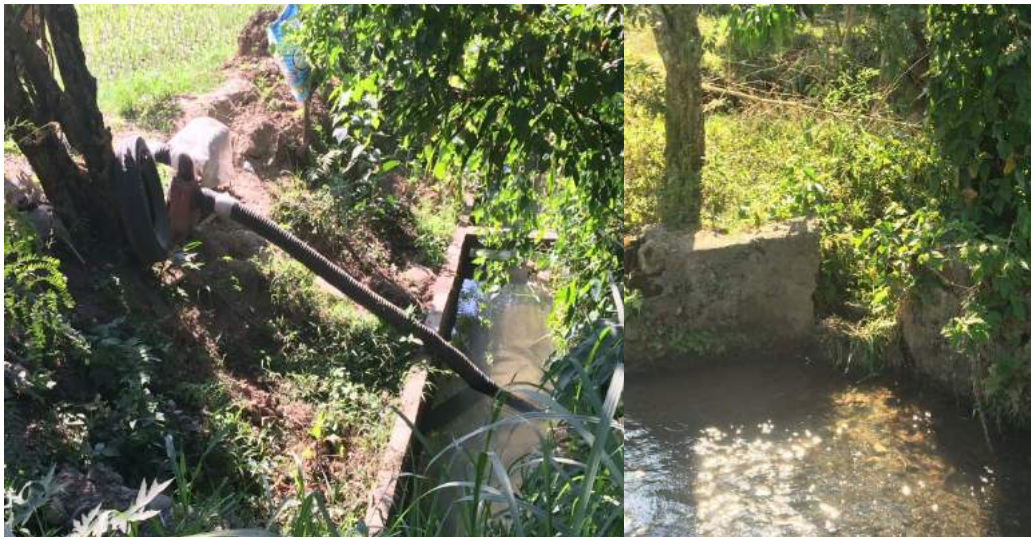
Figure 1A-75. Portions of the main canal with illegal pumps (left) and improvised lateral turnouts (right)
