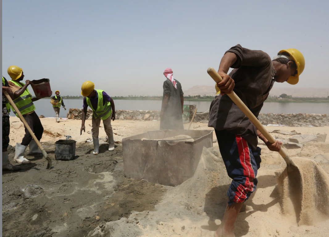
Egypt Emergency Labor Intensive project aims at creating short term employment opportunities for unemployed unskilled and semi skilled workers and provide access to basic infrastructure services. These construction workers are building stronger river banks along the Nile river to protect it from erosion. Photo: Dominic Chavez/World Bank
