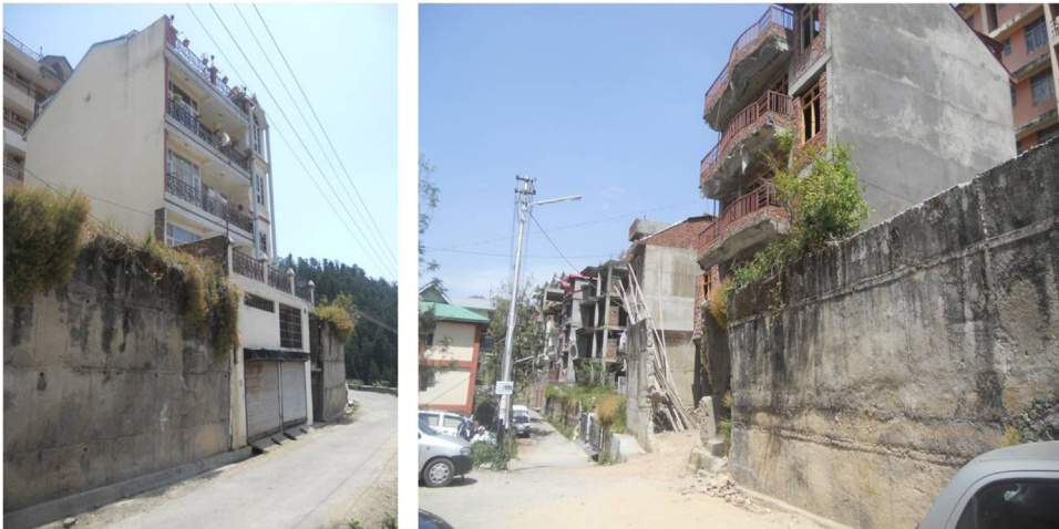
Fig. 15. Addition of extra storey after demolition of retaining walls in New Shimla.
