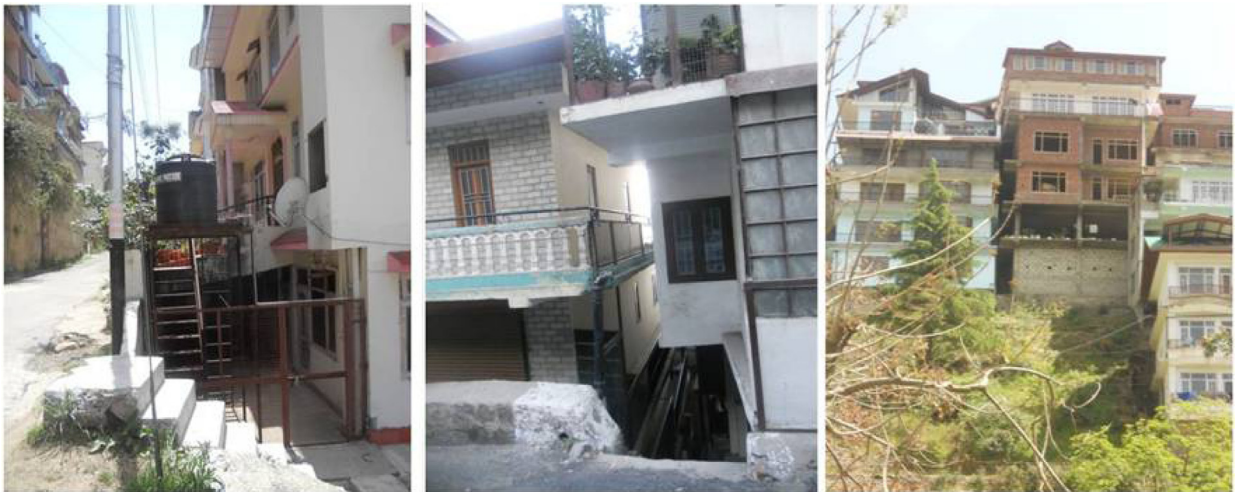
Fig. 14. Insufficient setbacks around multistoried buildings in New Shimla Township.
