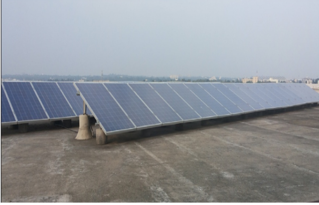
Fig. 2. View of 11.2 kWp rooftop grid interactive solar PV system.
