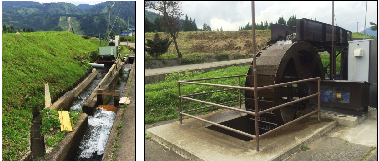
Photo 1 (left) and 2 (right): Installation examples of generator in Itoshiro, Japan Source: photos taken by Ohno, 2014
